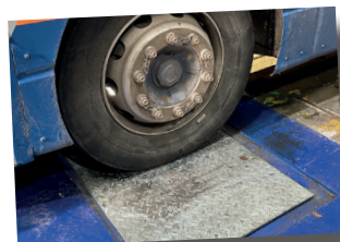
New shaker plates installed in our MOT bay
