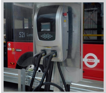
Charging point: One of 34 charging points for the new electric bus fleet.
